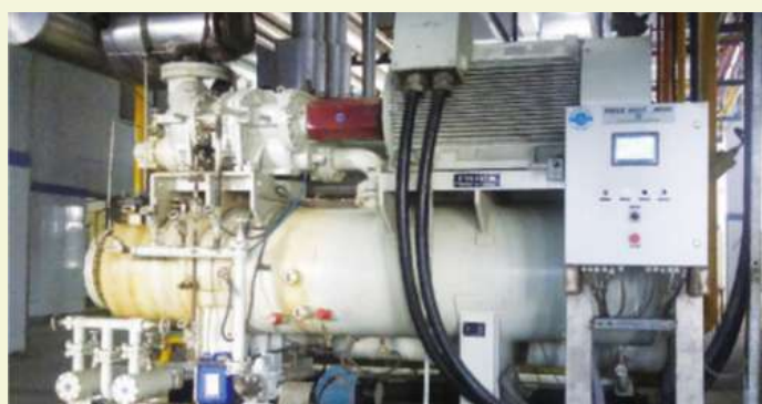
Air compressor at refrigeration plant
