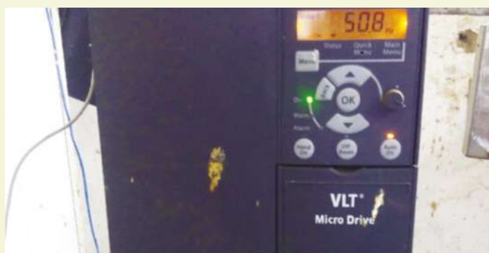
VFD installation at refrigeration compressor motor
